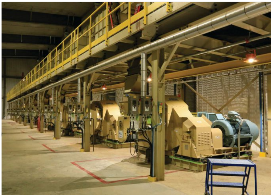
The new facility features 10 Andritz LM26 II pelletizing machines as part of a $92-million investment.
